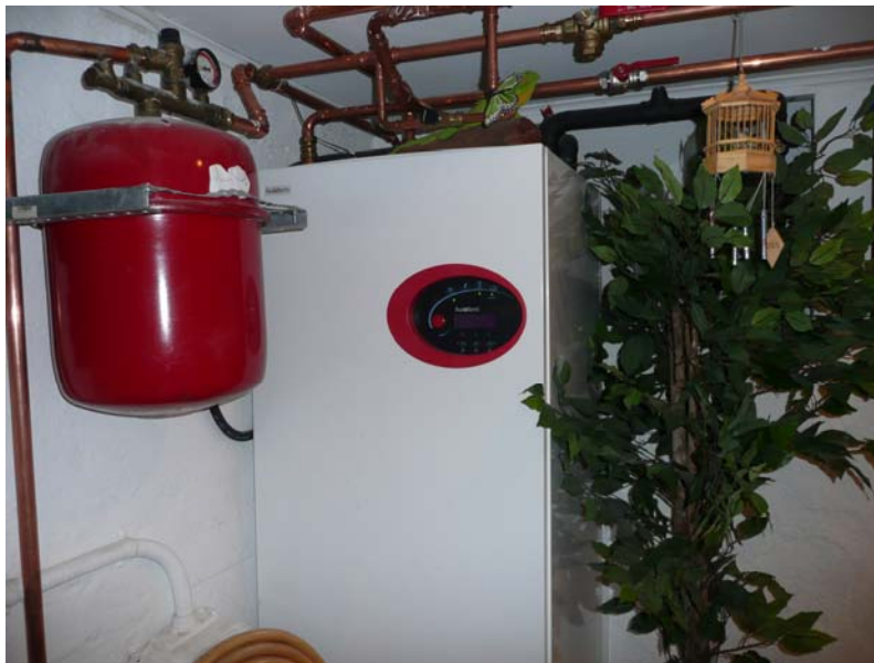
Central heating in the basement
